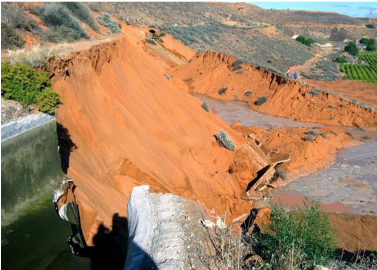
Figure 3.12 | Lower Olifants Canal break in 2015 (IOL, 2015)
