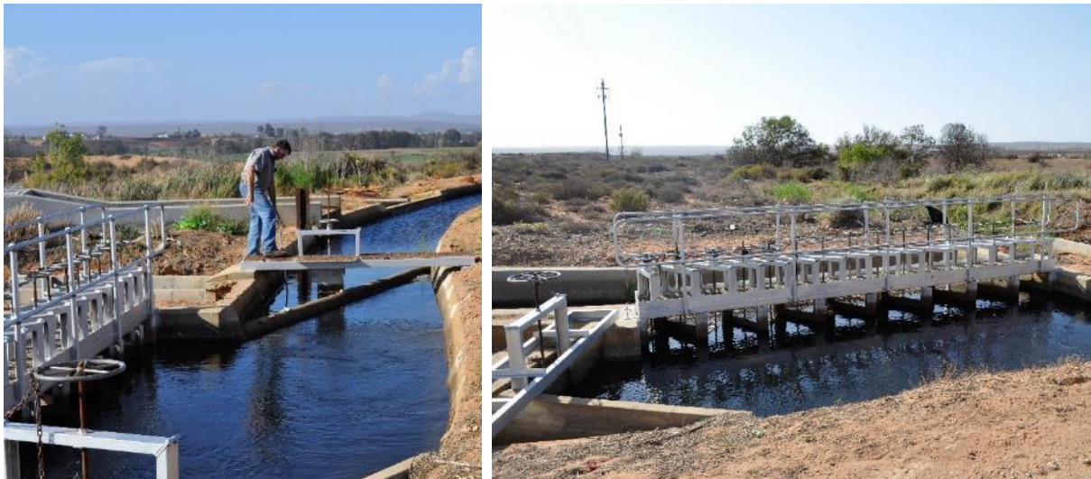
Figure 3.18 | Sluice gates installed near the Ebenhaeser balancing dam
