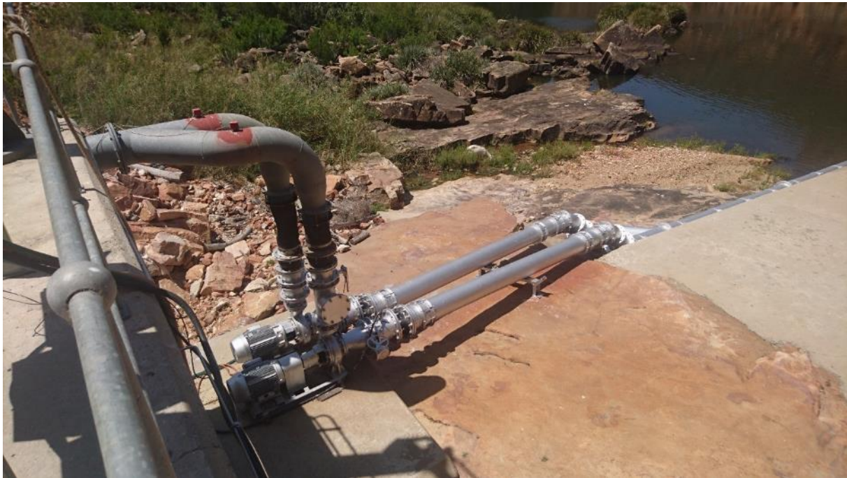
Figure 3.8 | Pumping system installed at Bulshoek Weir to recover leakage
